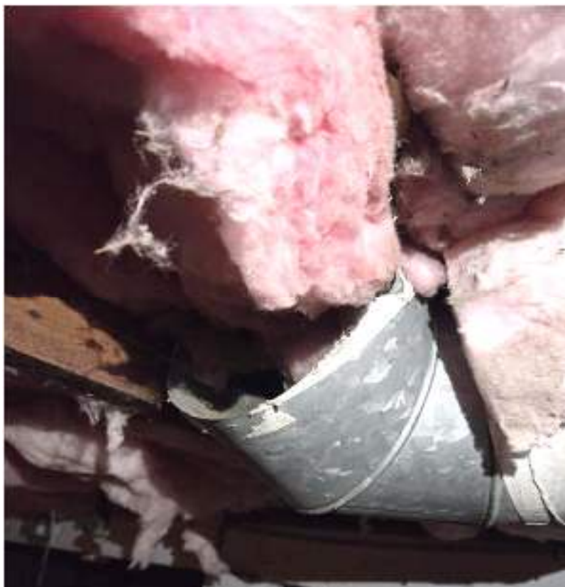
Photo 4: Sample: 03 ACM sealant tape on HVAC pipe
