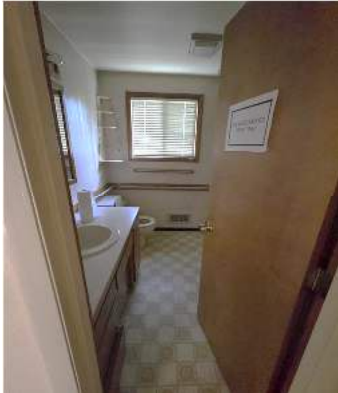
Photo 5: Sample 04 ACM vinyl sheet backing under vinyl flooring
