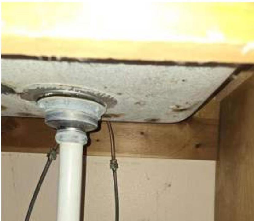
Photo 3: Sample 18: ACM White sink undercoat in utility room
