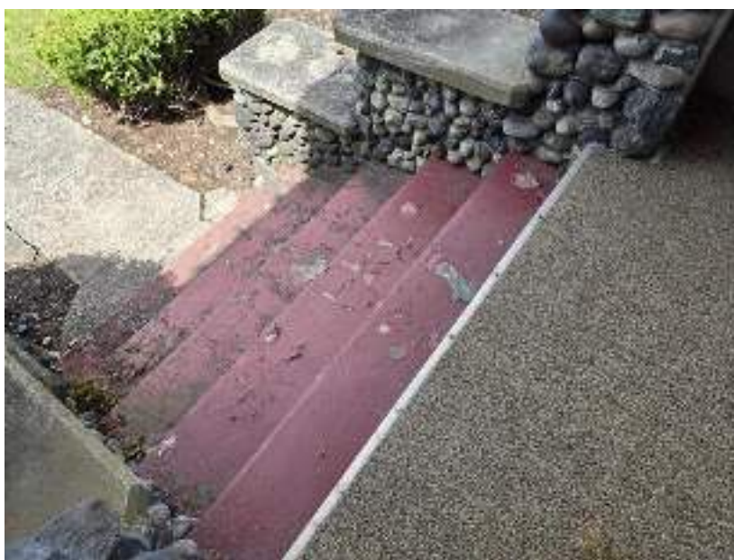
Photo 8: Sample L3 Lead-containing red paint on stairs ( 0.047% Lead )
