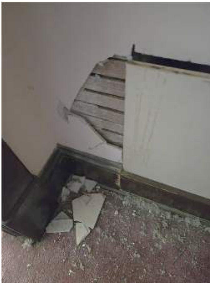
Photo shees Photo 9: Sample L11 Lead-containing pink paint of plaster walls ( 0.022% Lead )
